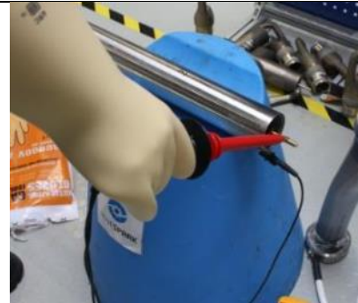
Use the HV probe from the multimeter to confirm the absence of voltage into the PSU
