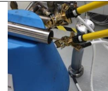
Using the sticks to short-circuit the asset.
