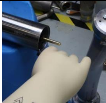
Using HV gloves, connect the HV probe's ground clip to the housing of the PSU
