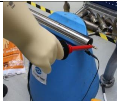
Use the HV probe from the multimeter to confirm the absence of voltage at the pin.
