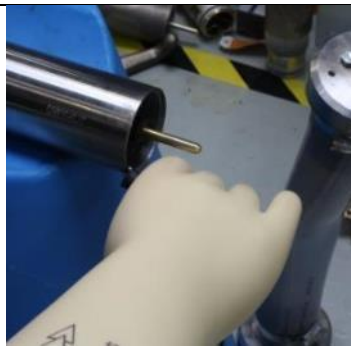
Using HV gloves, connect the HV probe's ground dolphin to the PSU housing.
