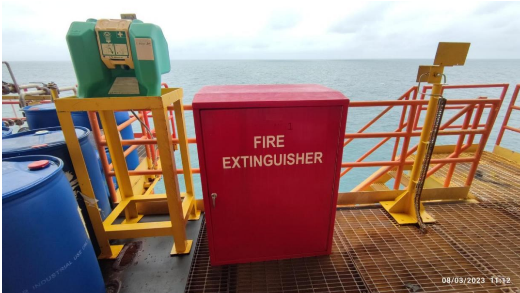
Fig: Fire extinguisher box at cellar deck.
