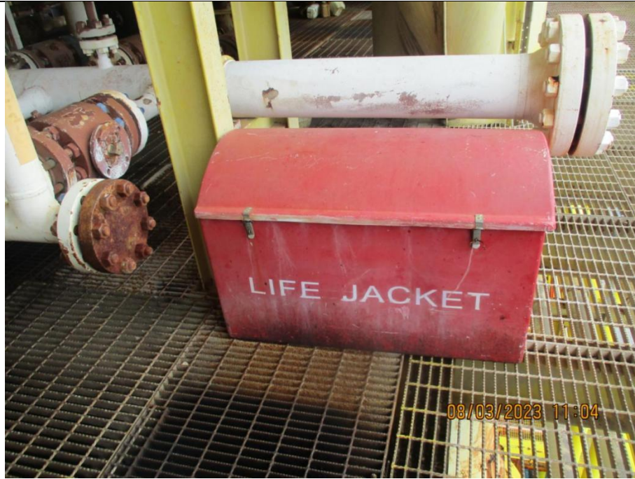
Fig: Life jacket box at cellar deck.
