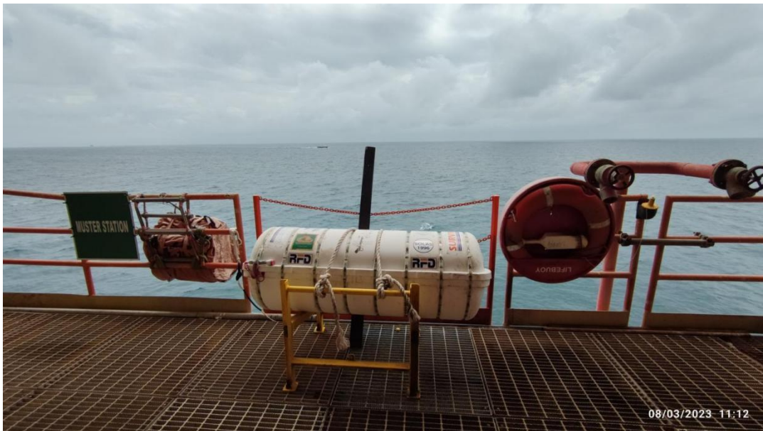
Fig: Liferaft 25pax, lifebouy & escape ladder at cellar deck.
