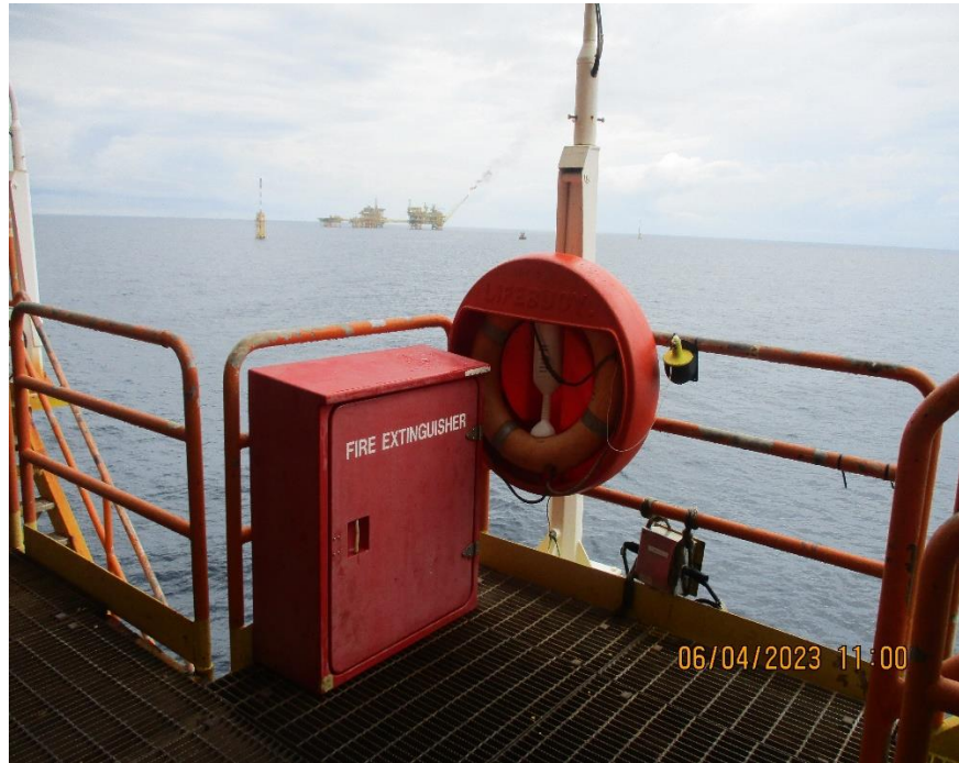
Fig: Fire extinguisher box at cellar deck.
