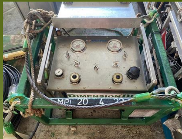
Single Well Control Panel
