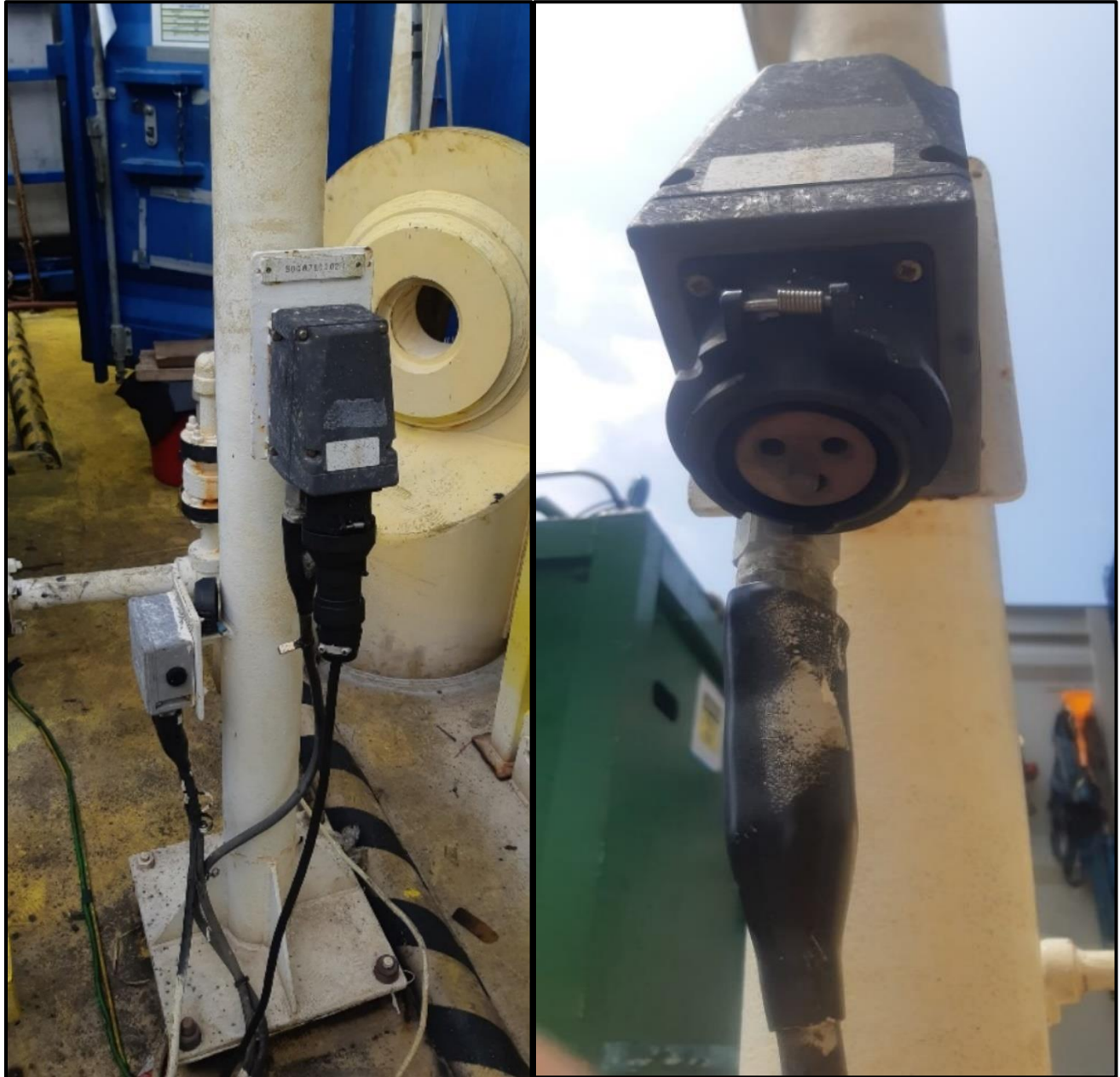
Fig: Single Phase 240/220 VAC Power Source on Main Deck.
