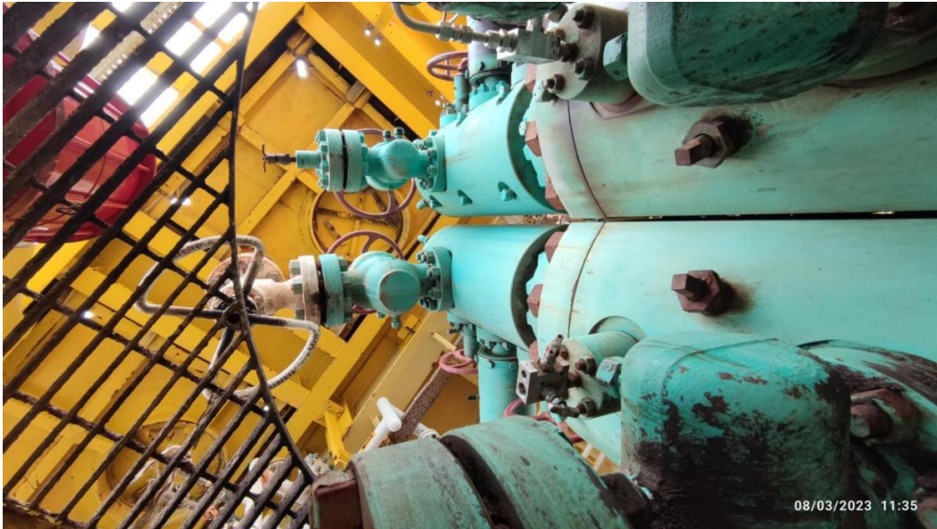
Fig: X-max tree well By-220 & By-222 view from lower deck to hatch cover above.
