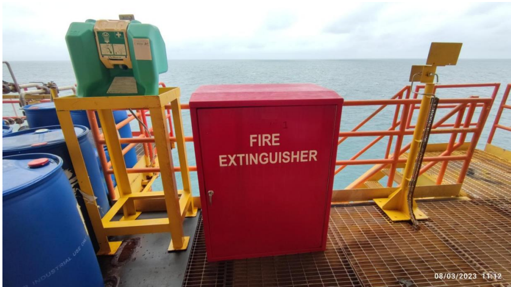
Fig: Fire extinguisher box at cellar deck.
