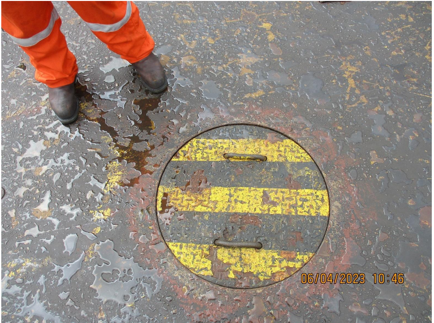
Fig: View from hatch cover to X-mas tree.
