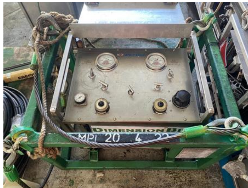
Single Well Control Panel
