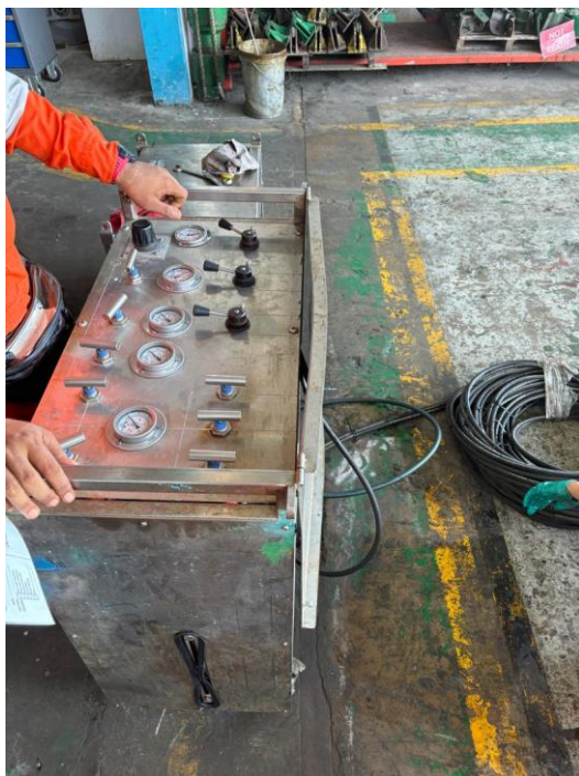
CONTROL PANEL (CP)
