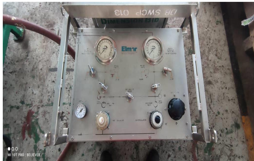
SINGLE WELL CONTROL PANEL (SCWP)
