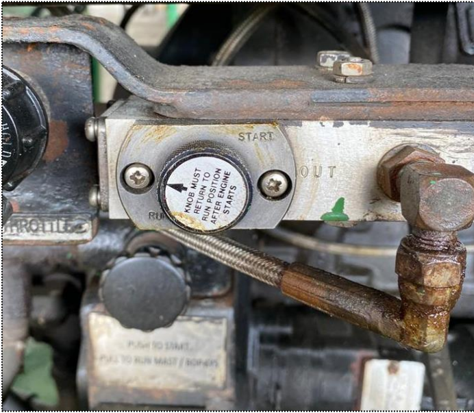
Diesel cut off valve
