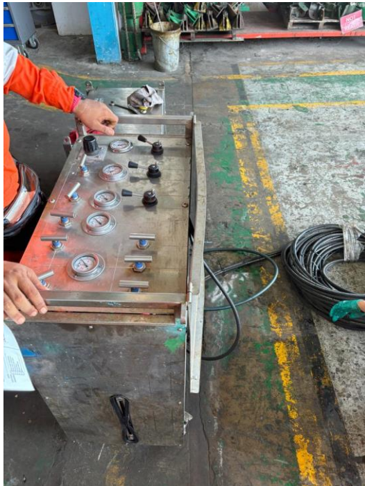
CONTROL PANEL (CP)
