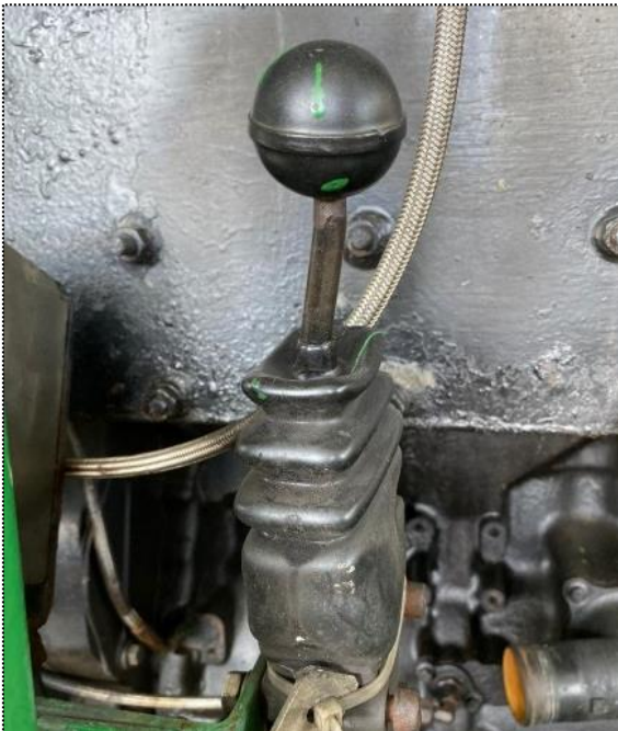
Inlet overspeed shut down valve
