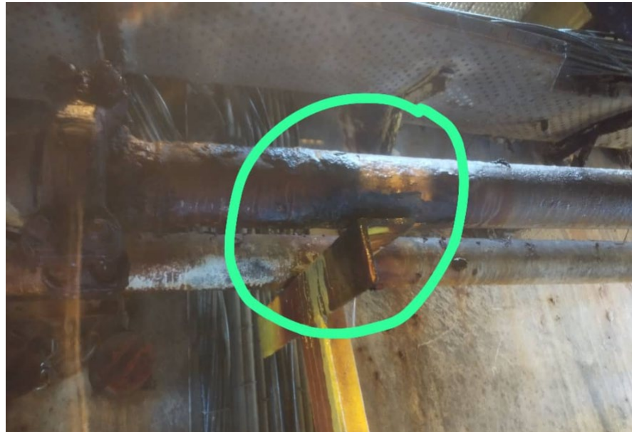
Dulang D5S injection flow line pinhole leak located below WH grating
